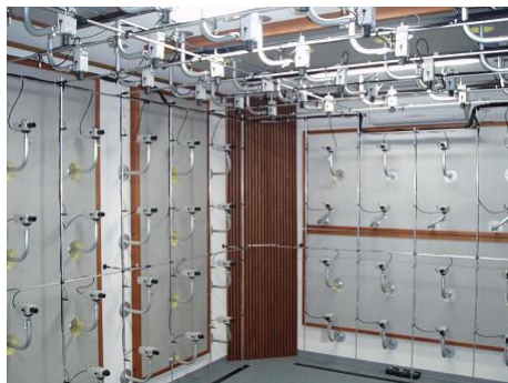
Figure 3: Image of surrounding microphone array room [7].
